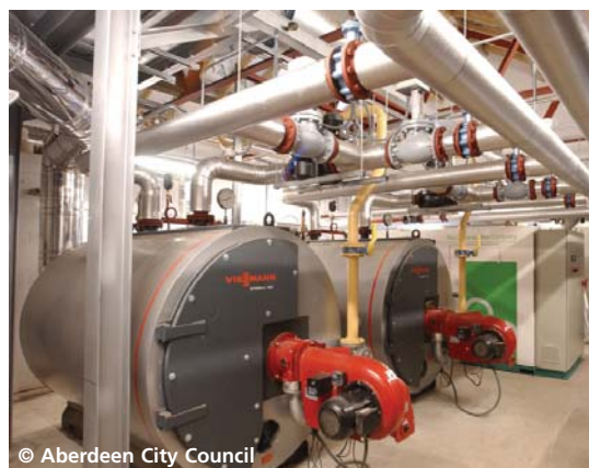
Figure 2: The energy centre at Stockethill
